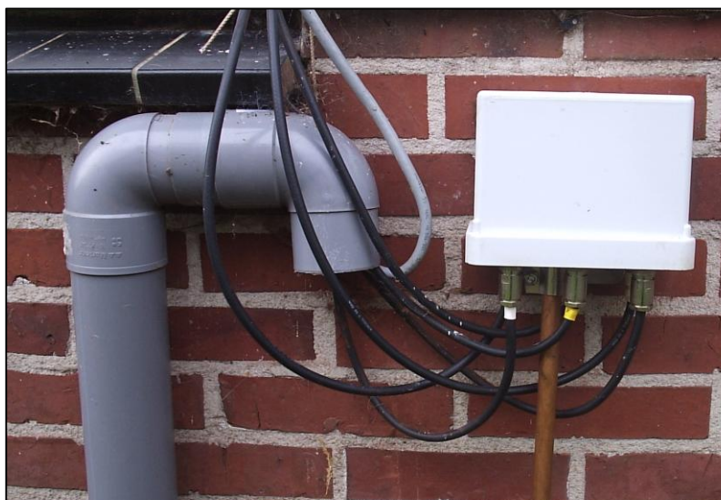
The lightning arrester box mounted above one of the 4m copper ground pipes.
